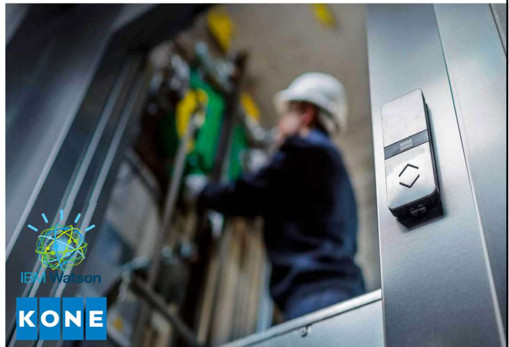
Lifts and Escalators [13]
